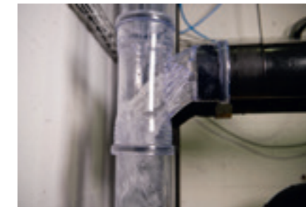
... and the identical result is visible in real conditions in the Geberit drainage tower, which forms part of the test laboratory.
